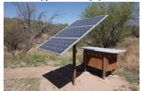
Cottage solar system
